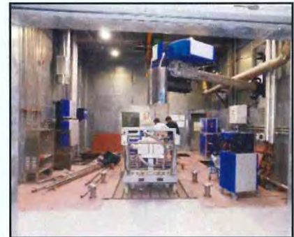
Engine Test Cell
